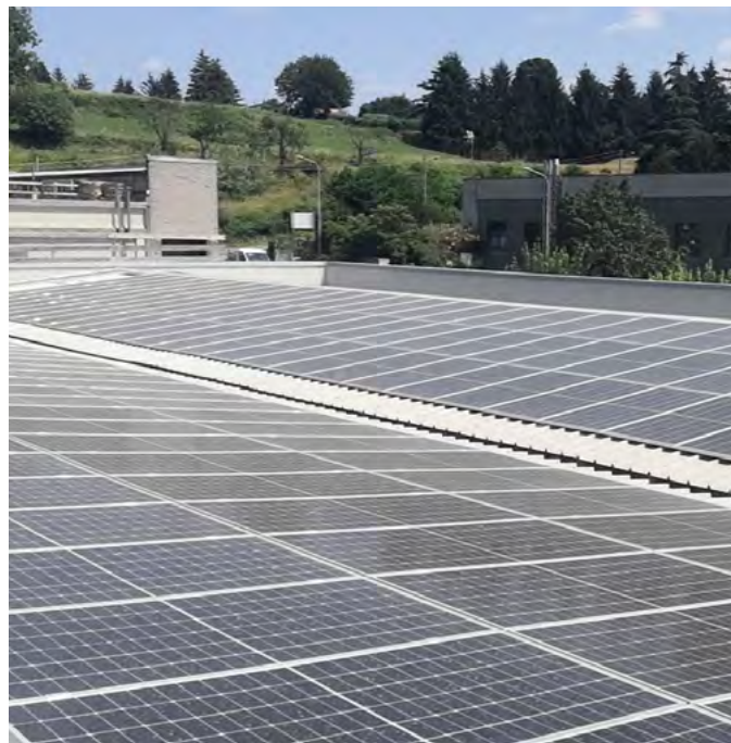
Photovoltaic installation in Grassobbio (BG)
