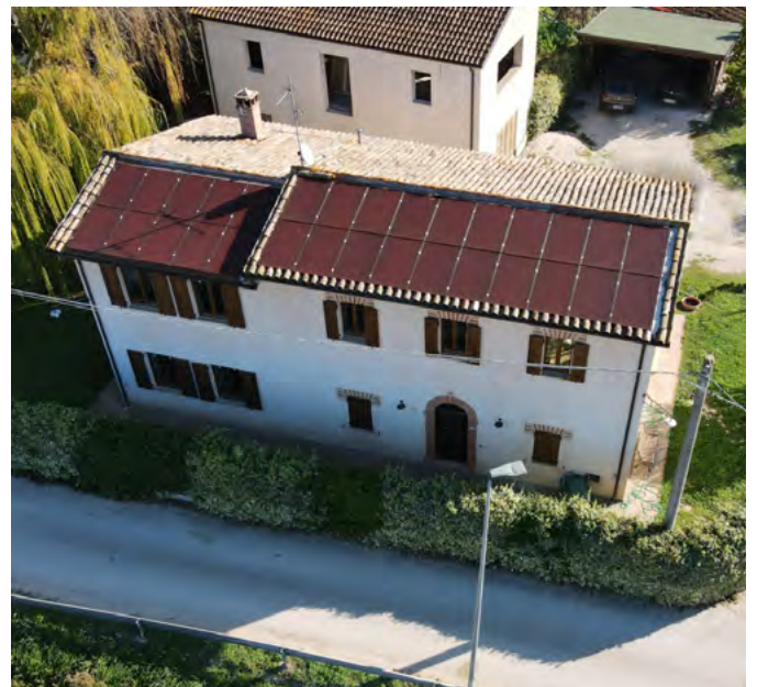
Colored PV plant in Campello sul Clitunno (UNESCO site)
