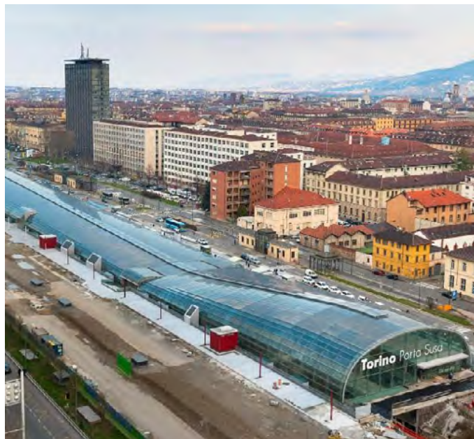
Glass-glass PV plant in st. Porta Susa, Torino.
